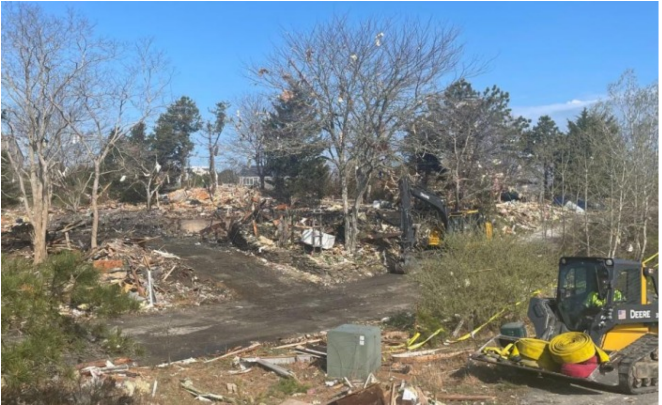
Truro Fire Department photo.
